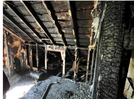
Figure 6.26 The damage sustained by the roof structure due to the fire.
