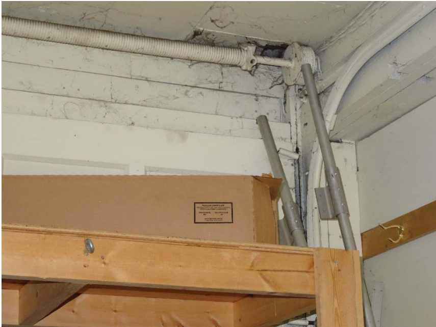
Original 3x2x12 beam inside the workshop wall in the ground floor; the beam is not connected to the 6x6 posts.
