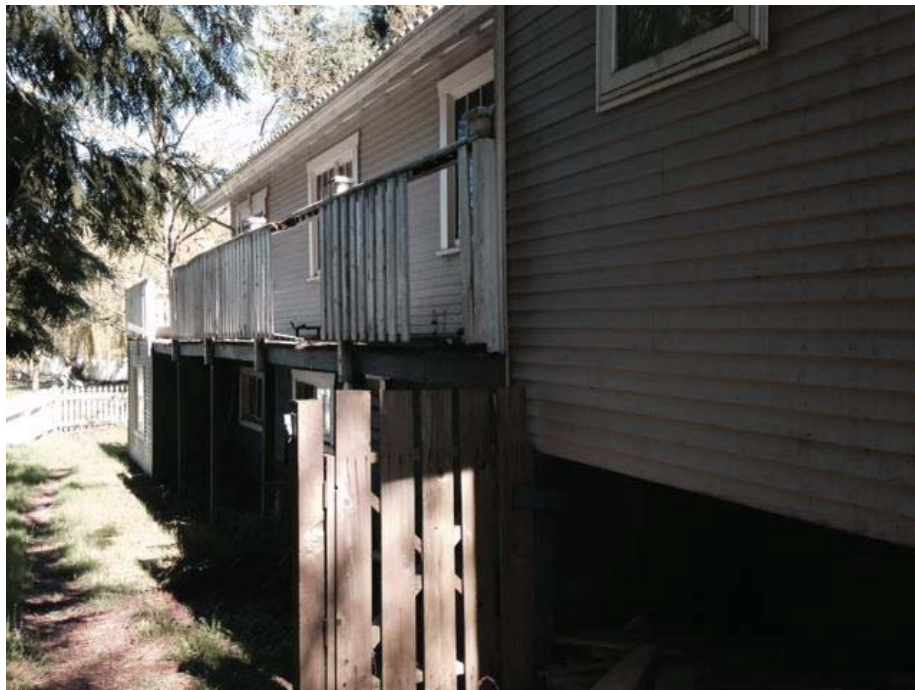
West elevation of the Lee House revealing unsympathetic extended side porch with wood railings.
