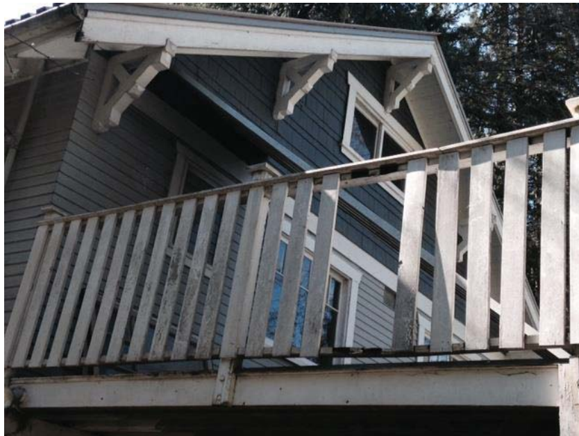
Lapped wood siding, twin-coursed shingles and triangular eave brackets under the gable ends. Unsympathetic porch addition with railings in foreground to be removed.
