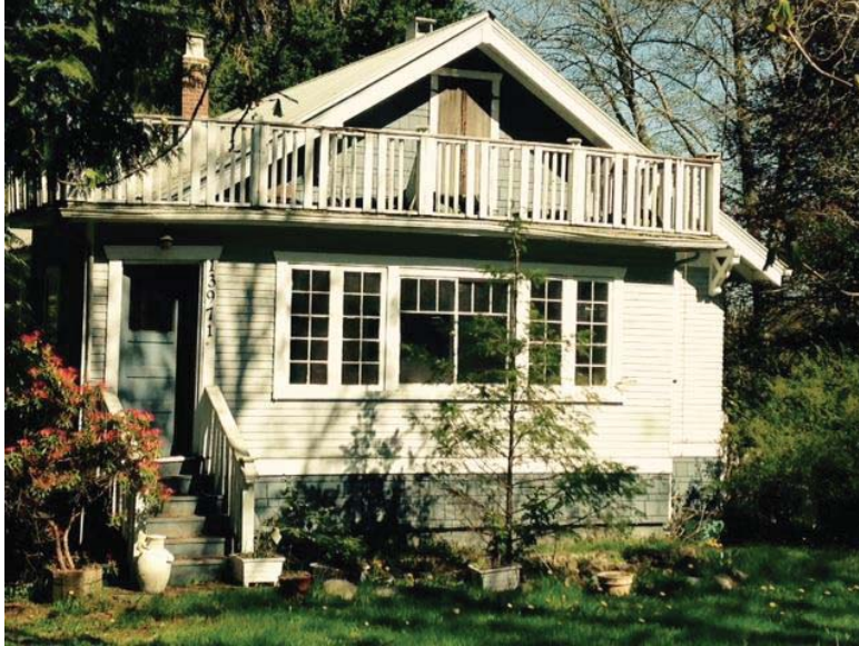
Front of Lee House showing evidence of a settling foundation
