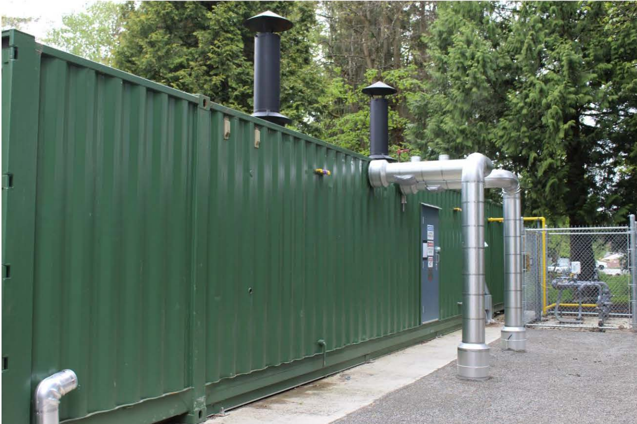
Temporary District Energy Facility at 10357-133 Street
