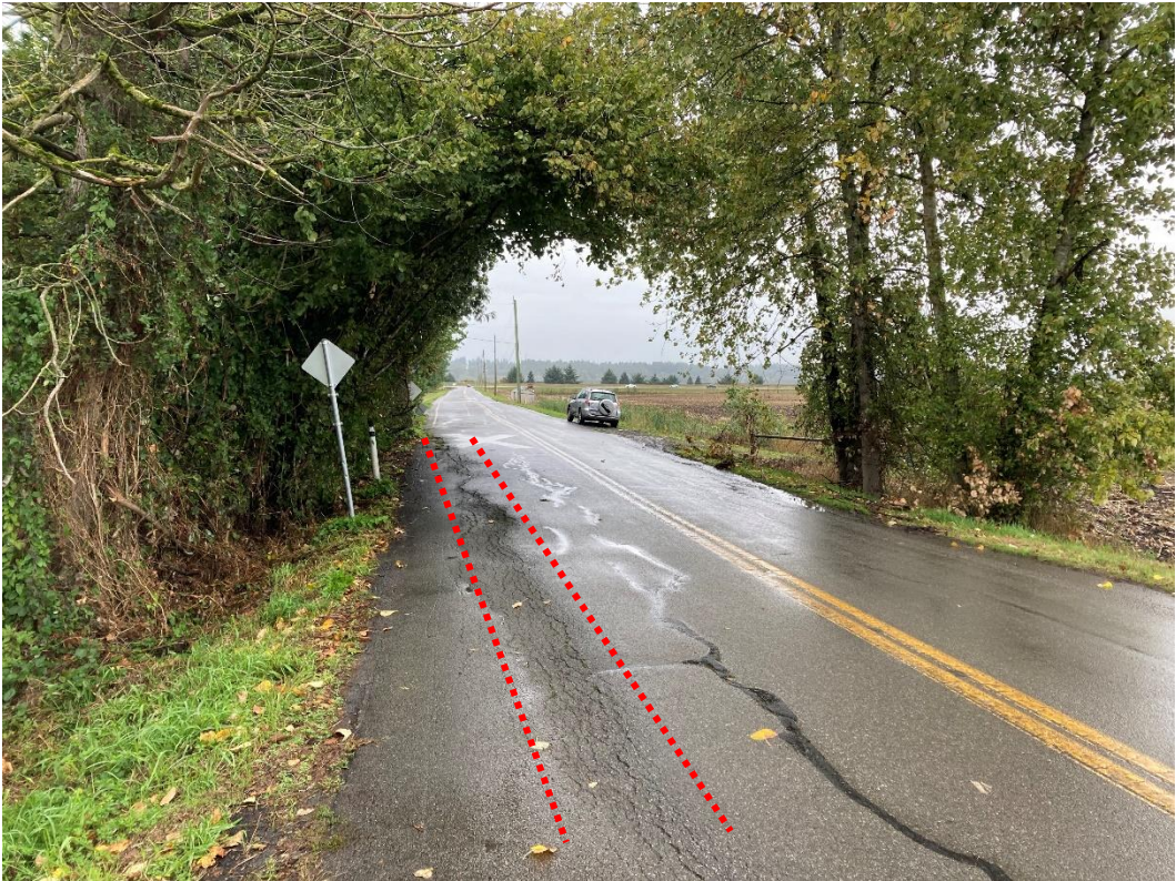
Photo 5 – Looking north at longitudinal cracking in SB lane about 35 m north of rail crossing.
