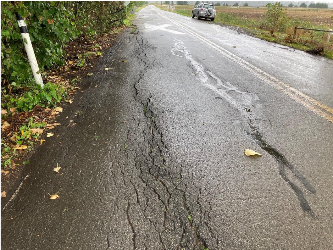
Photo 6 – Close up view of longitudinal cracking visible in Photo 5.
