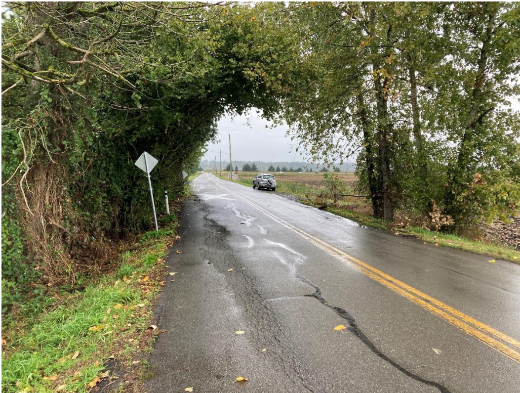
Photo 5 – Looking north at longitudinal cracking in SB lane about 35 m north of rail crossing.
