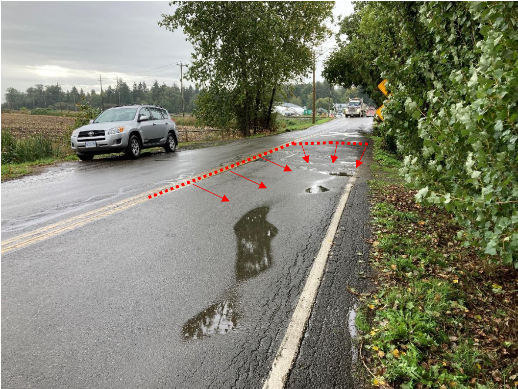
Photo 3 – Looking south at depression in front of south driveway
