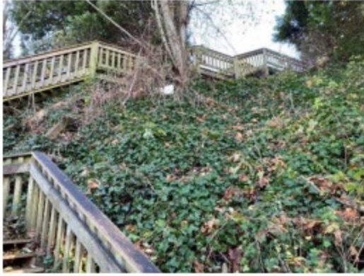
Photo 33 – Minor landslide North of stairs
