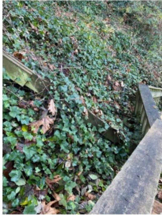
Photo 34 – Soil pushed against railing
