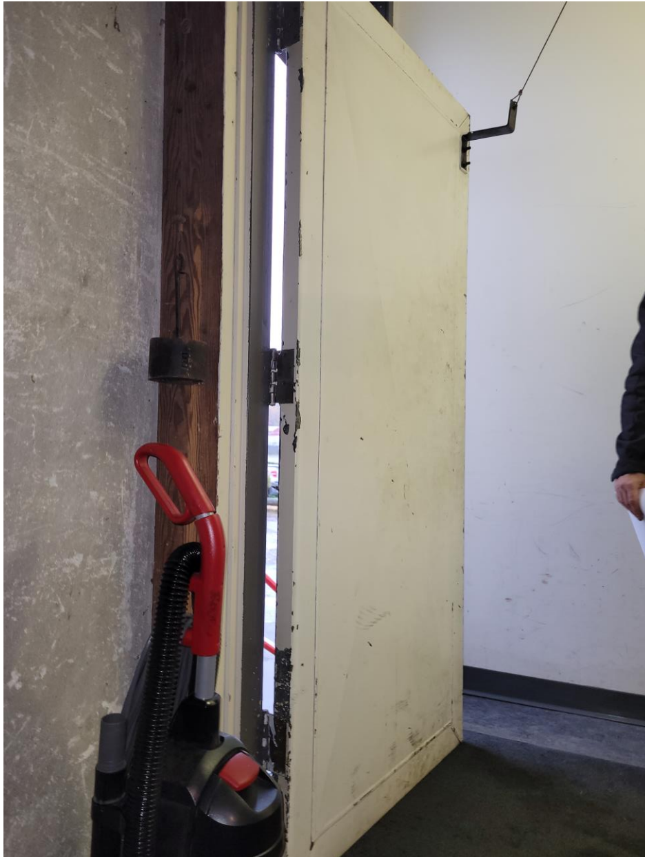
Photo # 3 – Fire door with presumed asbestos-containing lining & lead-based paint coatings. Lead-based paint on plaster is pictured on the Hallway wall
