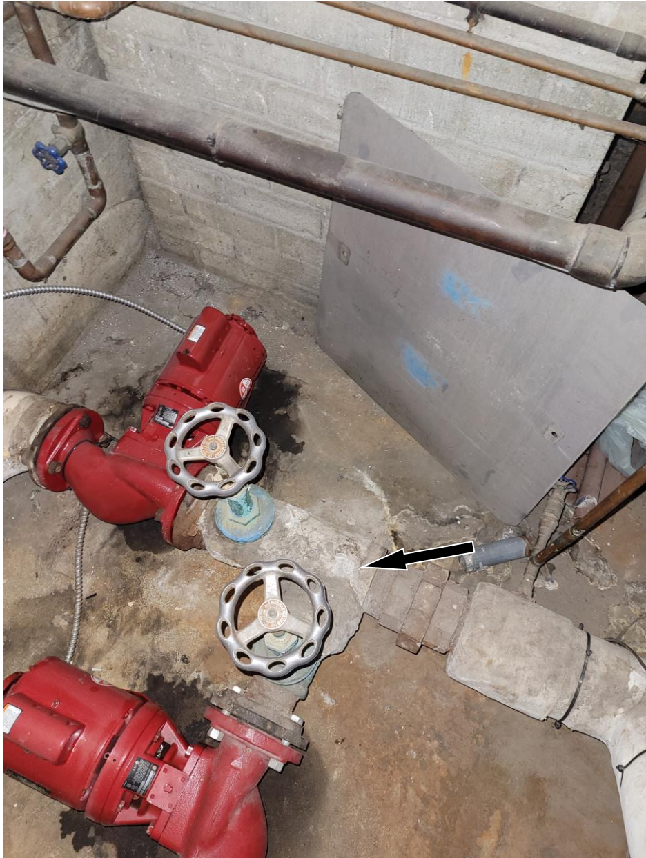
Photo # 2 – Asbestos-containing parging cement
