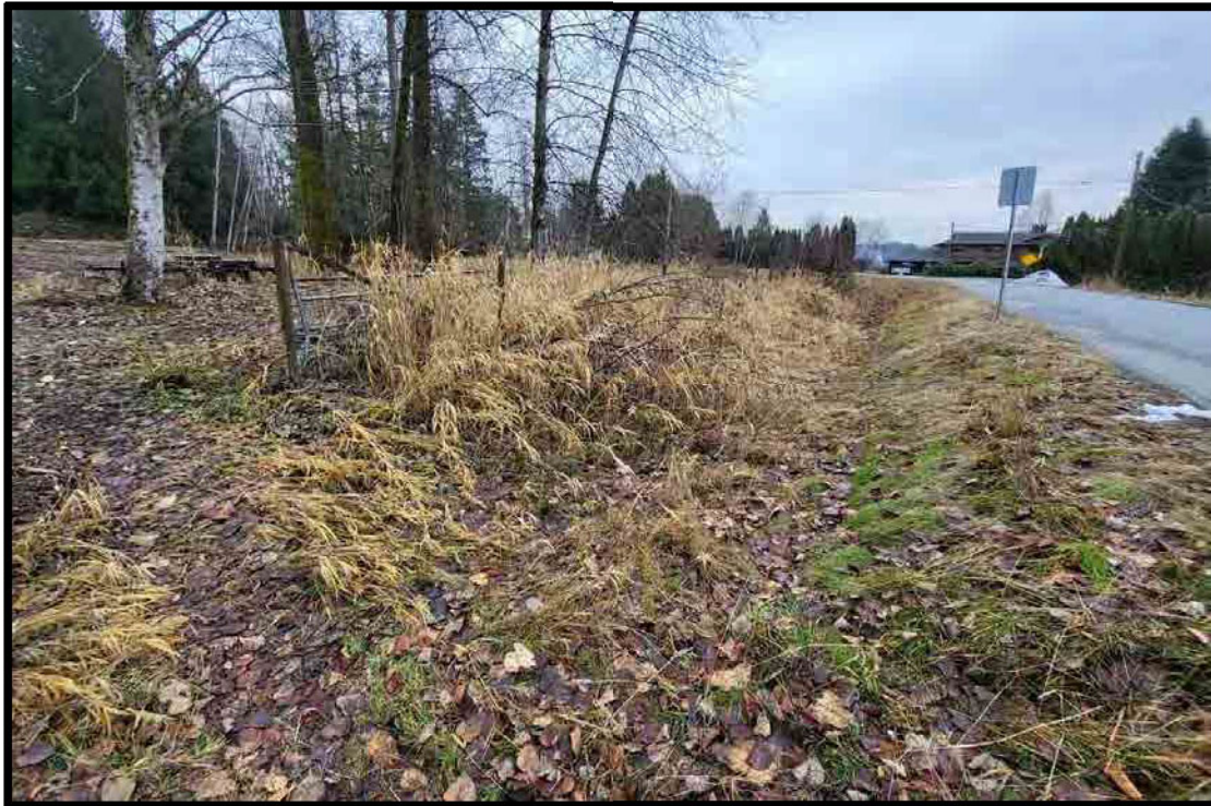
Photograph B15. South (downstream) view of the Bothwell Drive ditch, taken near a vehicle crossing for the western property (December 13, 2022).
