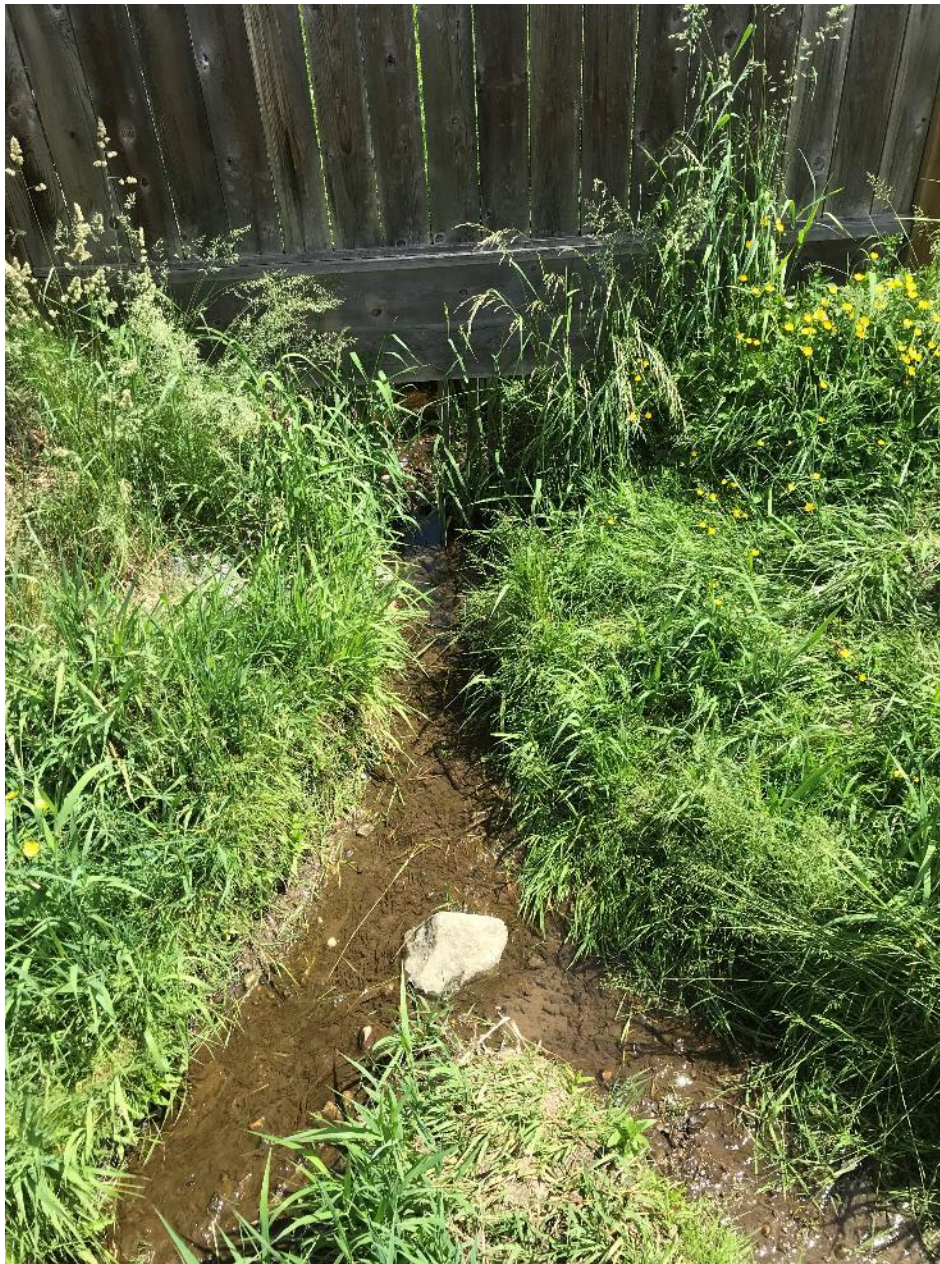
Photograph 6. View of WC2 facing east. This location is where the watercourse leaves the neighbouring property and flows through two pipes under a pedestrian path before flowing across the utility ROW to the west of the subject properties.
