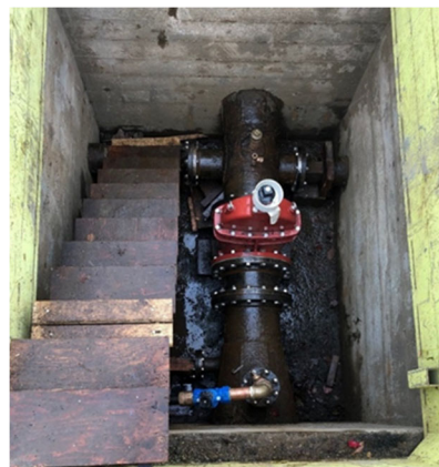
Water Valve Chamber
