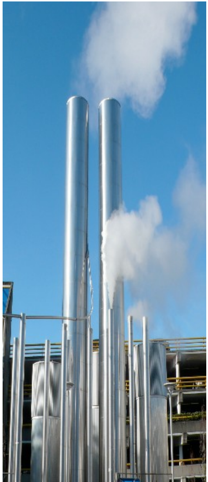
Vertical stacks of the Boiler Plant below.
