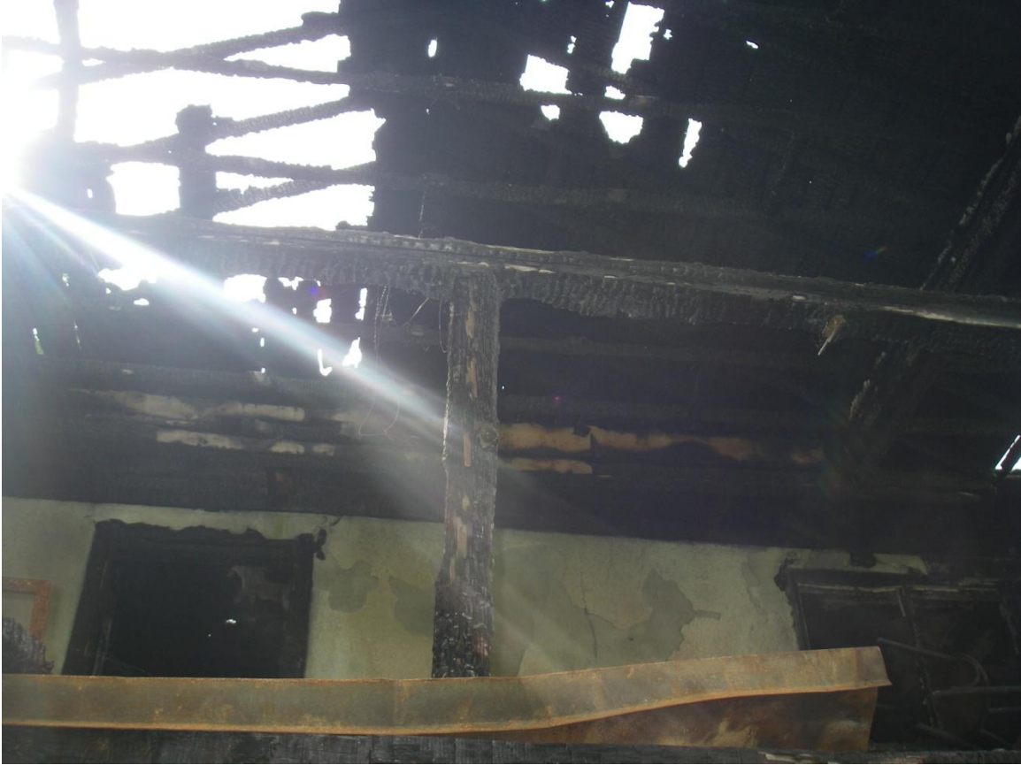
Photograph looking up at the railing and roof of the balcony at the back of the Structure
