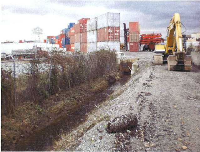
Photo 1: Drainage ditch southeast of the southeast corner of #11678 130 th Street looking west.
