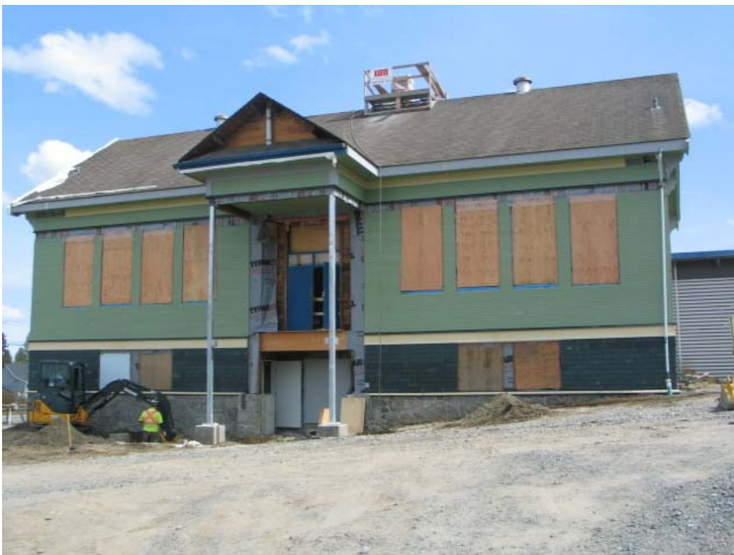
April 12, 2011 – Building enclosure removed, siding installed and restored. Window openings awaiting heritage window replacement
