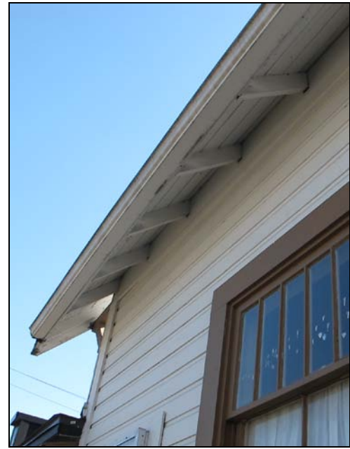
Exposed rafter tails
