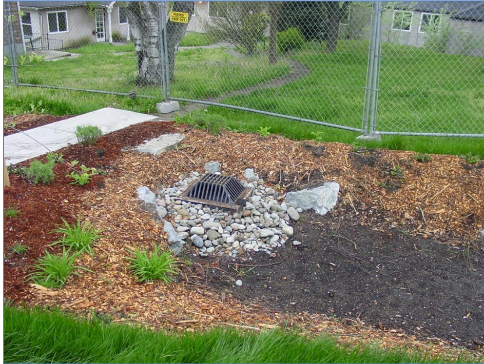
Typical bioswale overflow structure (prior to final vegetation planting)
