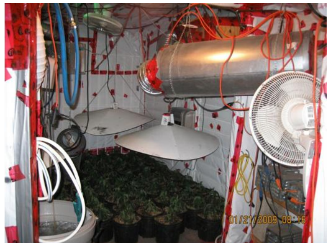
Scenes from medical grow operations in Surrey, B.C. Top: electrical safety hazards for work performed without permit or inspection. Middle: signs of mould and excessive moisture, as well as electrical safety issues. Bottom: various electrical and fire hazard issues.
