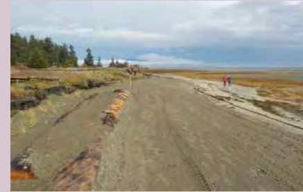
Expanded edge protects from storm surge and accommodates trails and other uses. Image courtesy of BC Parks
