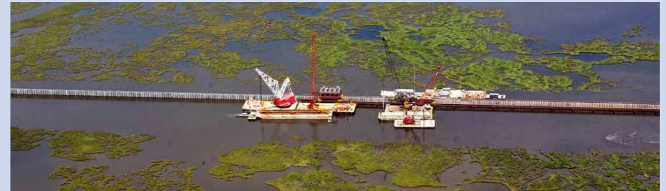
Louisiana surge barrier CC-by, Team New Orleans US Army Corps of Engineers
