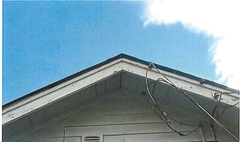
Figure 72: Exposed underside of roof decking
