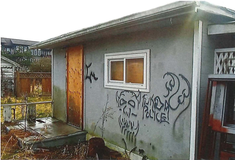
Figure 91: Plywood addition with PVC slider window
