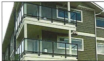
PONDER COATED ALUMINUM GUARDRAILS WITH TEMPERED GLAZING PANELS BLACK ALUMINUM WITH CLEAR TEMPERED GLAZING ELEVATIONS FINISH SCHEDULE NO. 7
