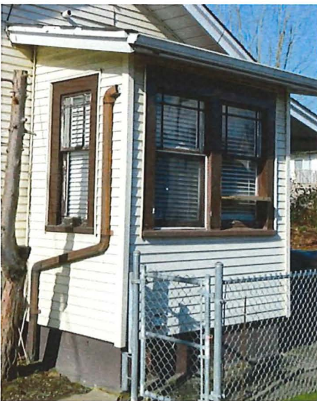
Figure 22: Disconnected eaves trough at dining nook
