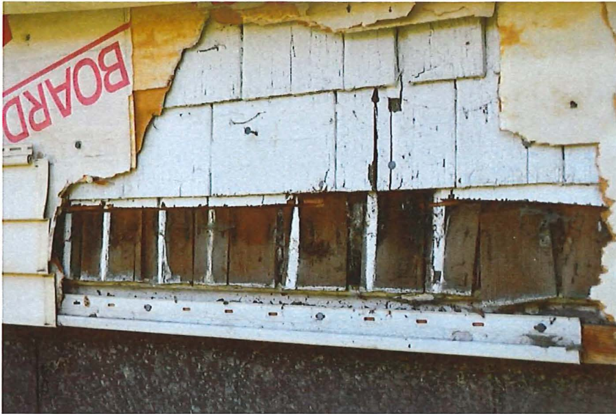
Figure 25: Painted cedar shingles behind vinyl siding and unpainted shingles behind
