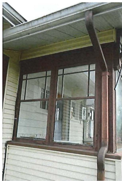
Figure 23: Eaves trough at southwest corner of front porch
