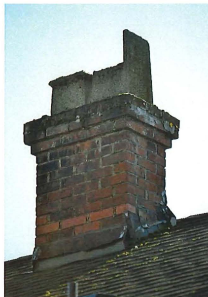
Figure 53: Exposed chimney shaft viewed from the backyard
