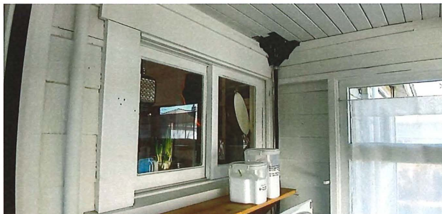
Figure 32: Interior of back porch with kitchen window on the left and cedar shingles on the wall
