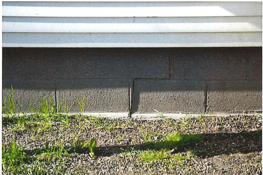
Figure 19: Disjointed concrete block
