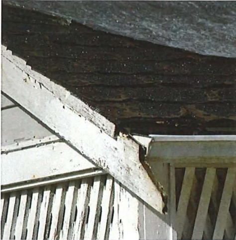
Figure 71: Tar paper on top of asphalt shingles
