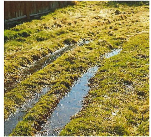
Figure 67: Ponding on the grounds of the cottage
