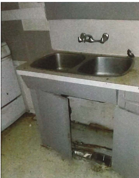
Figure 93: Rotten floor under kitchen sink
