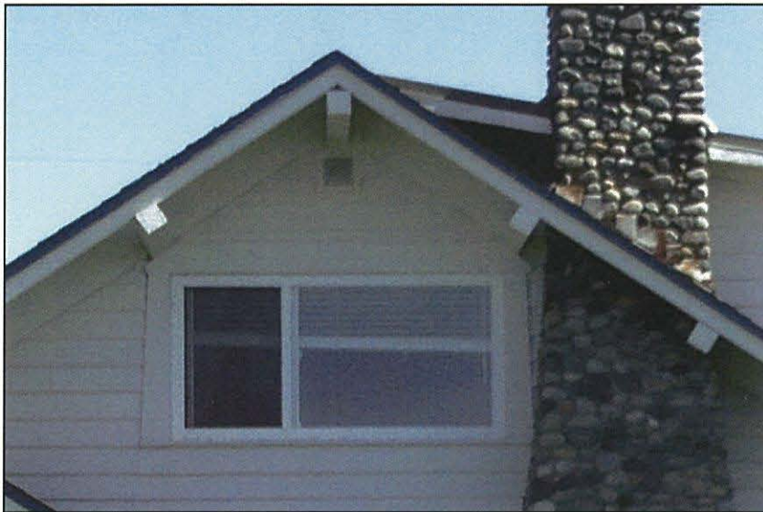
Photo 15: West gable end. Note poor condition chimney step flashing, exposed ends of roof purlins, window trim design & vinyl-framed window in an altered opening.
