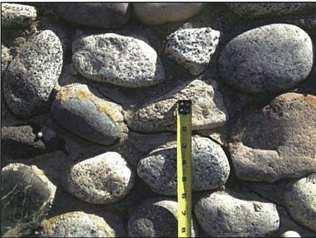
Photo 14: Typ. cracking of later mortar repairs.
