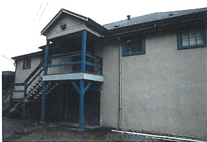
Front (west) façade of Tynehead School; note the absence of the basement level windows. The faint impression of a window beneath the stucco can be seen in the bottom right-hand corner of this photo.
