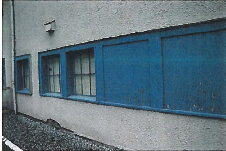
Basement level of Tynehead School, south façade, boarded-up basement windows.
