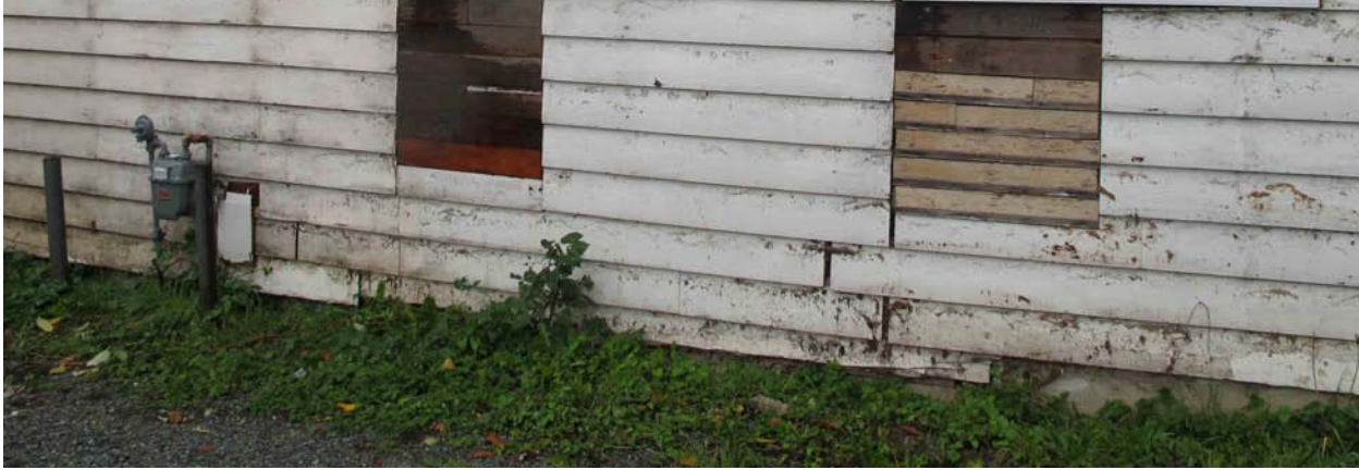
East façade of the building showing the foundation at the lower right corner
