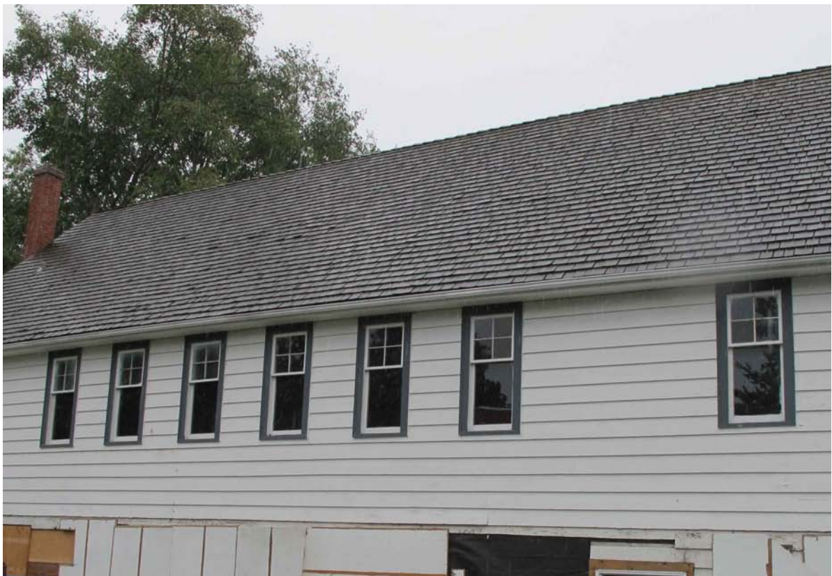
Original historic windows of the Seventh Day Adventist Church on the west façade of the second storey
