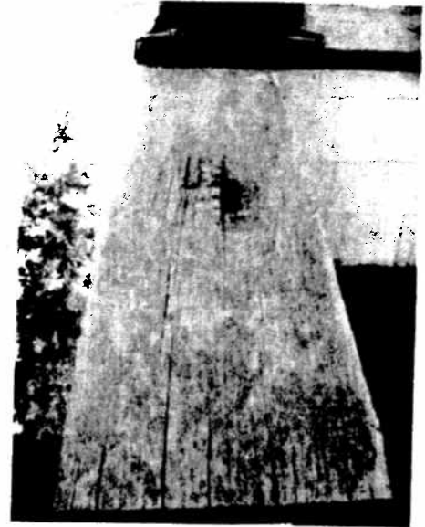
PHOTO 26: Mould damaged balustrade sill
