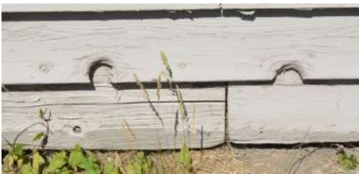
Figure 38: Rough wood siding boards with fallen knots
