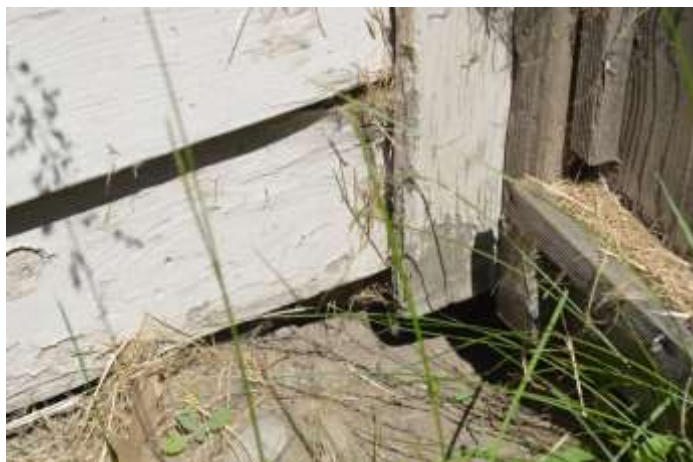
Figure 16: Exposed siding at grade next fence
