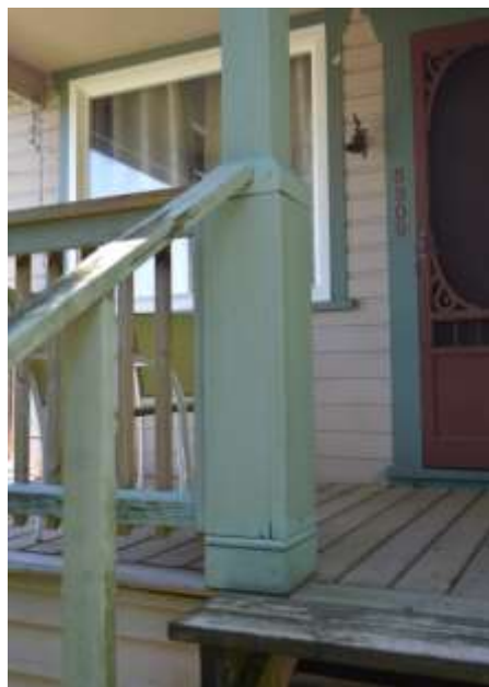
Figure 30: Porch post base and front door trim
