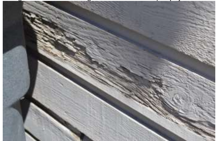
Figure 43: Damaged reversed board & batten siding at staircase enclosure
