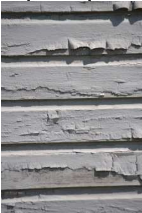
Figure 44: Paint peeling off cover lap siding
