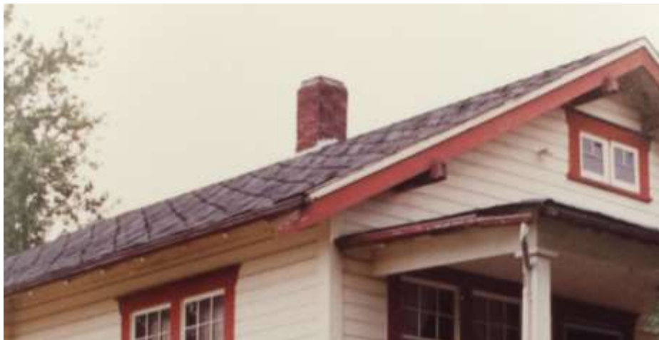
Figure 77: Former chimney positioned on the roof ridge approximately in the middle of the house
