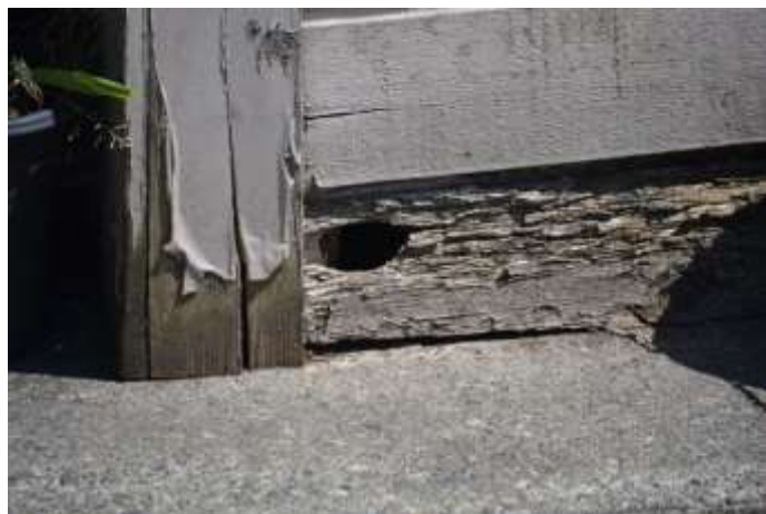
Figure 15: Exposed siding at grade
