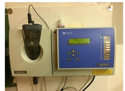
Online chlorine analyzer at Whalley Pump Station
