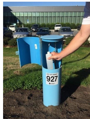
Water Sampling Station at 148 Street
