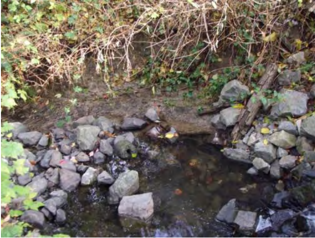
Photo 1. Minor erosion downstream of outfall near 76A Ave.
