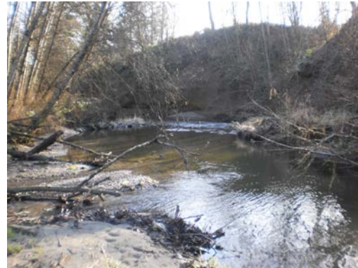
Photo: Bear Creek Erosion at 148 th Street.
