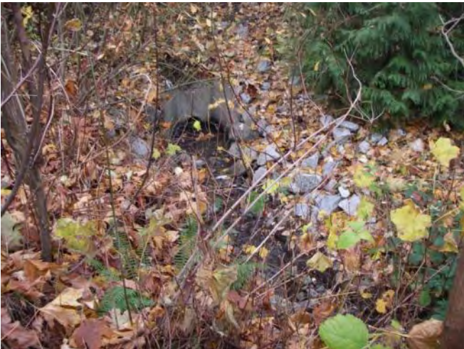
Photo 9. Small unmapped storm outfall originating from trailer park.
