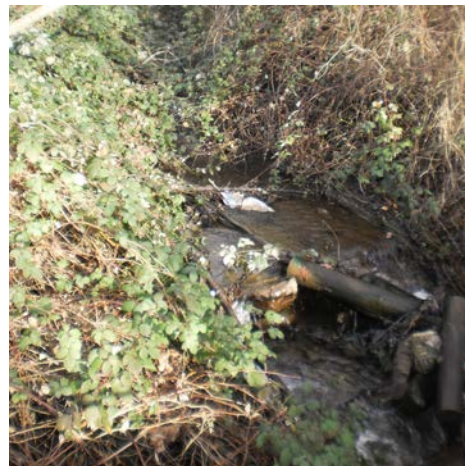
Photo: King Creek at 90 th Avenue showing some signs of debris and erosion. Extensive blackberry also noted.
