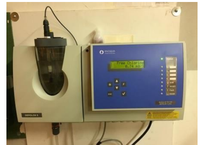
Online chlorine analyzer at Whalley Pump Station
