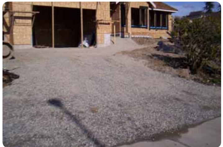
This angle of the same construction site shows that the builder has installed a gravel access pad for managed site access. The installed perimeter controls further act to restrict vehicles to this site access point, which that helps to keep the roads clean.
