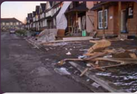
This single family construction site shows no ESC management on-site. Perimeter controls, surface protection, a gravel access pad and regular road sweeping should be implemented to prevent stormwater pollution.
