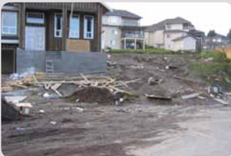
The site shows significant soil migration from the work area onto the road. No BMP's are present on this site and the road drainage is located under the material in front of the stockpile located in the middle of the image.
