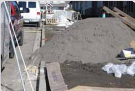
This image shows poor placement of an uncovered stockpile, no site perimeter controls, no surface erosion protection and dirt accumulated on the road and gutter.
