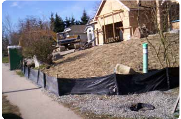
The above single family construction site shows a complete approach to site ESC management. There are perimeter controls, surface protection using straw, CB protection and the paved surfaces are clean.
