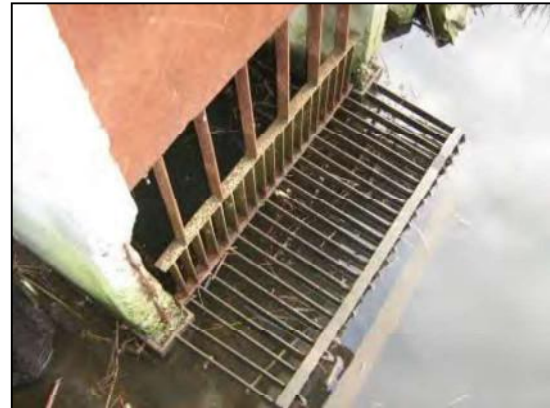
Pump station intake and trash rack
