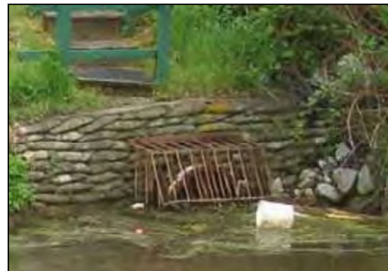
Flood box inlet
