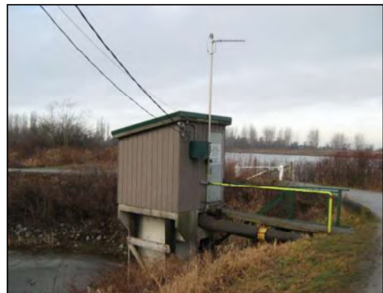
Maple Drainage Pump Station
