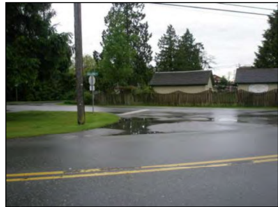
Surface ponding at Sullivan Street and Kidd Road
