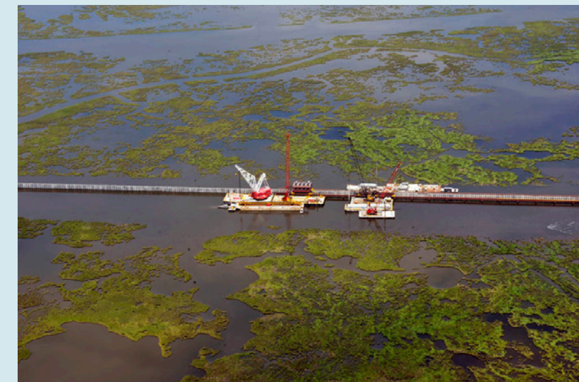
Louisiana surge barrier under construction CC-by, Team New Orleans US Army Corps of Engineers, flickr.com
